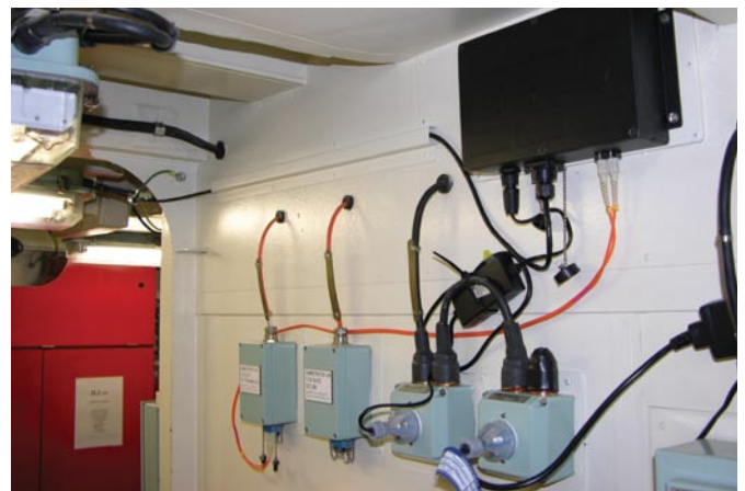
Condition-Based Monitoring system apparatus mounted on board HMAS Ballarat.
