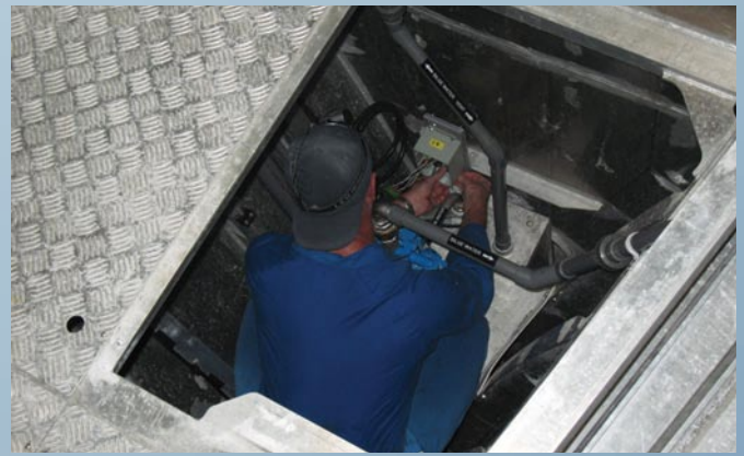
DSTO structural monitoring network sensor node being installed on Navy patrol boat, HMAS Glenelg.
